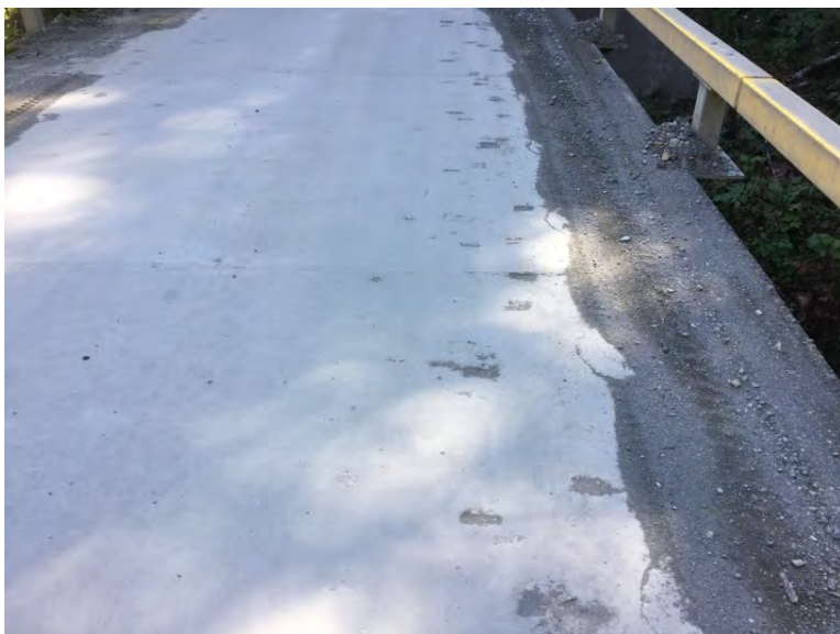
Minor damage to deck from track equipment
